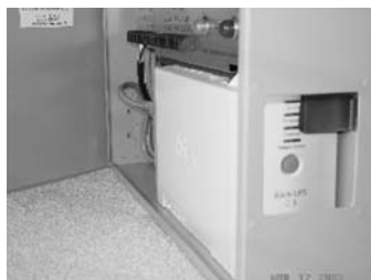
Battery System Status Indicators
